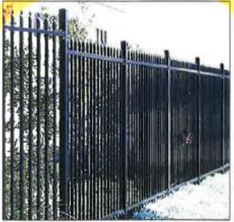
1.8m high black powder coated palisade metal fence to boundary to meet DA conditions and comply with AS 1926.1 and NSW Government Child Care Planning Guideline - 2017.
